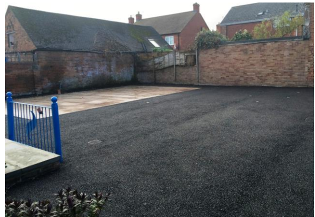
The new surface showing the footprint for the new marine engineering building
